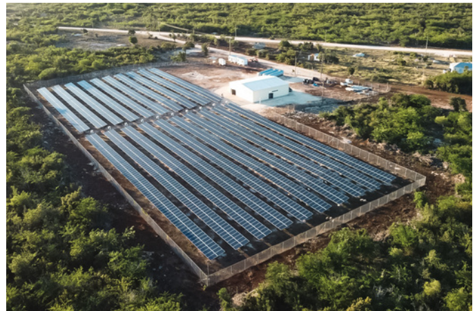
Solar power plant in Barbuda
