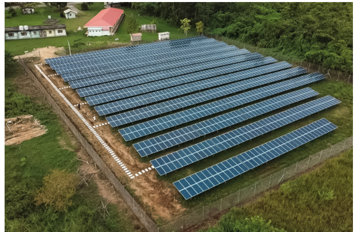
Solar power plant in Belize
